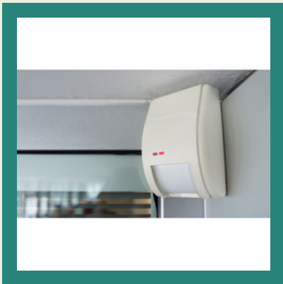
Intruder Alarm System
